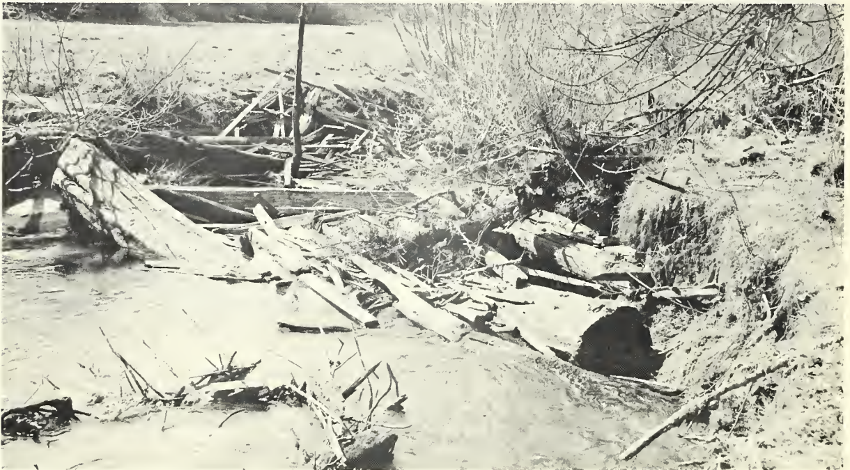
Photo 29.--Debris in Maple Creek should be removed so it will not cause bank erosion and overflow, 1964. SCS photo No. 7-1529-11
